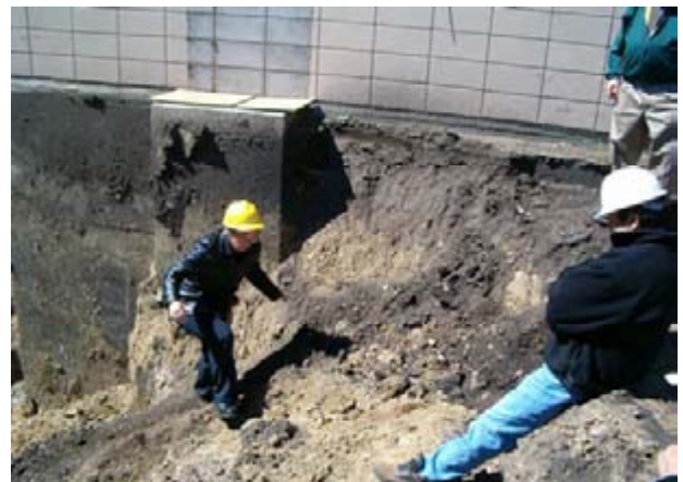
Preeceville Health Services Manager, Joanne Bodnar, does her part in site inspection.
